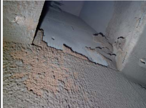
Figure 2. Example of dirty boiler heating surfaces, TPP Kakanj, BiH
