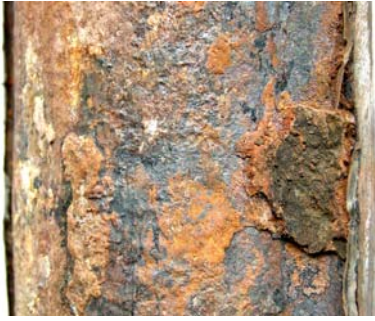
Figure 4 Tube fire side outer surface
