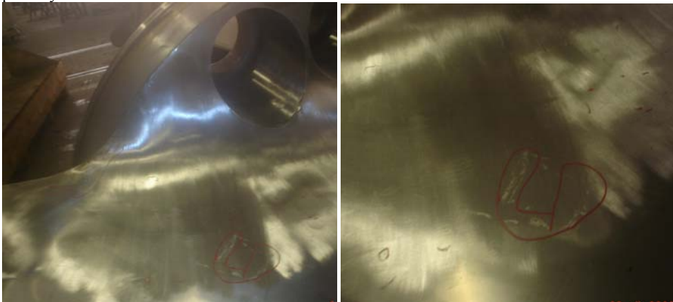
Figure 1. Shoulder blades of turbine with detected places for repairing
