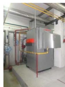
Figure 5. View on the new condensing boiler
