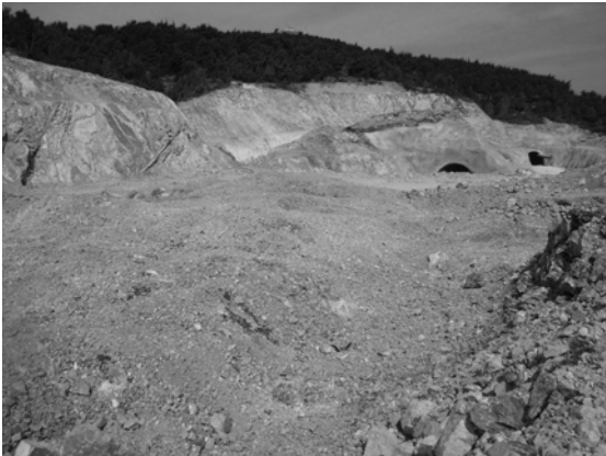
Figure 2. Terrain on the area of the highway route and fragmentation of the blasted material.
