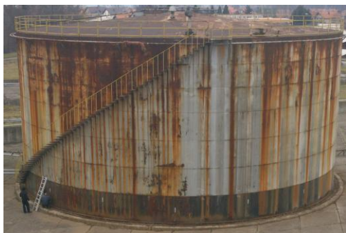
Appearance of complete tank corrosion (shell + roof)
