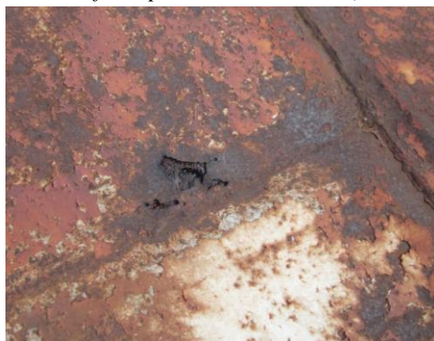
Pitting holes on roof plates close to bad welds
