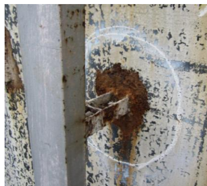
Pitting on shell support due to the bad welds
