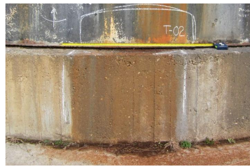
Corrosion products as sign of bottom perforation
